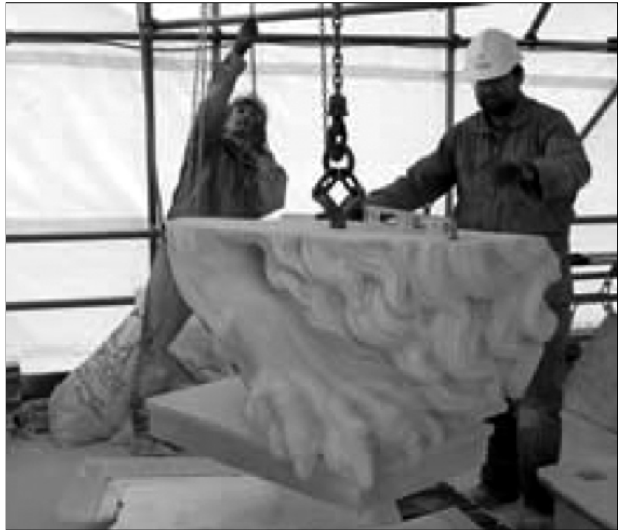
New carving is lifted using a hoist and carefully placed in position.
