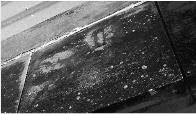
Indented Lewis Holes.
